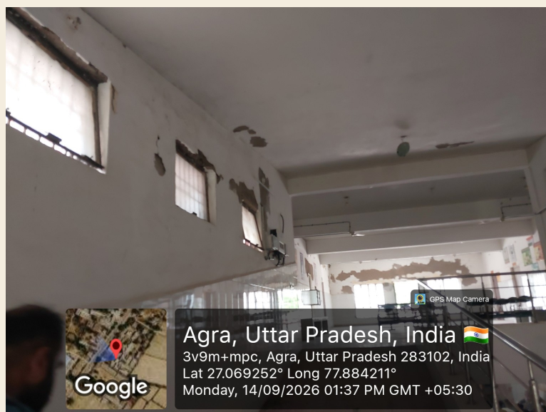
Larger internal section with widespread peeling/damaged wall finish.
