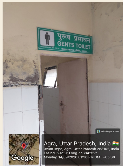
Public toilet entrance area showing visible dampness/ageing on wall surfaces.
