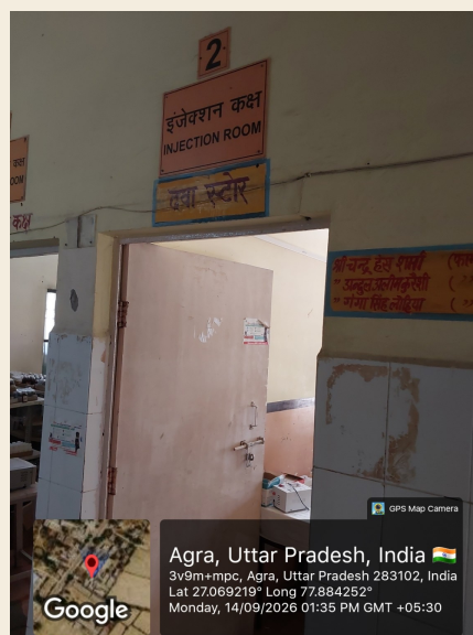
Injection room area with visible wear to doors, walls and finishes.
