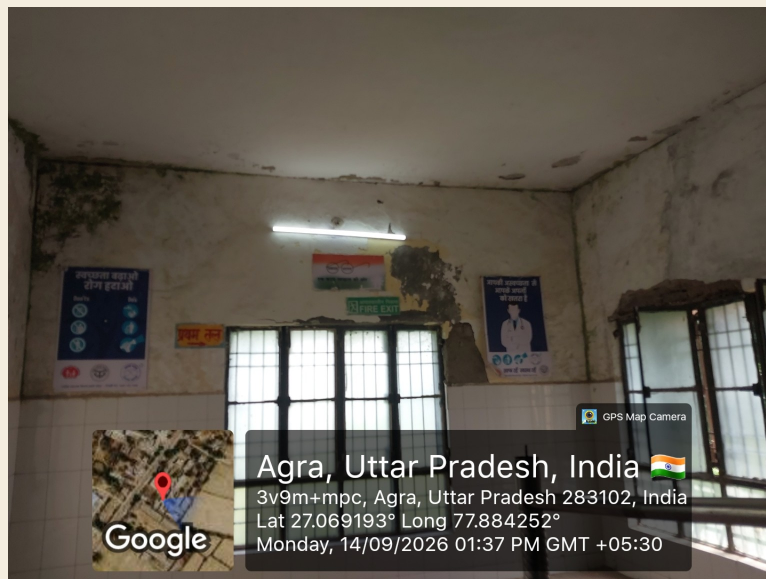
Ward/internal area showing deterioration and damaged wall/ceiling finishes.
